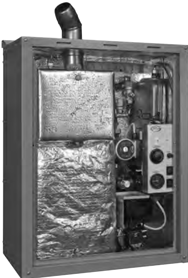
Figure 1-1: Boiler with front panel removed
